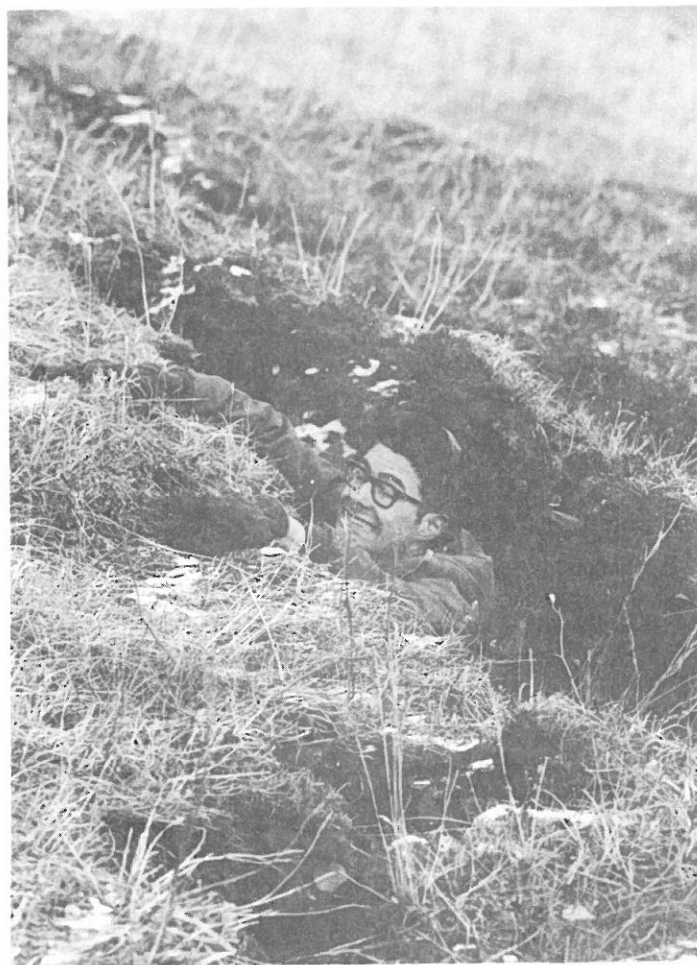
Above. Jim Peterson dramatizes the width and depth of fissures appearing in the slope above the slide area. Snowfall during the past week has obscured many of the smaller cracks. Photo by Randy Weisser
